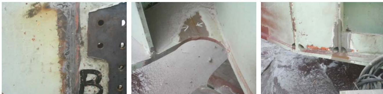
Slika 12. Oštećenja veznih nosača donje gradnje transportnog bagera Figure 12. Damaged connection beams in the excavator lower assembly.
