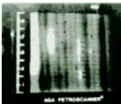
d. Povišena temperatura na tri reformerske cevi d. Elevated temperature of three reformer tubes.
