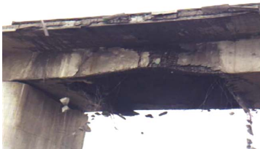
Slika 3. Most preko reke Morave oštećen tokom NATO bombardovanja Jugoslavije Figure 3. Bridge over river Morava damaged during NATO bombing of Yugoslavia.
