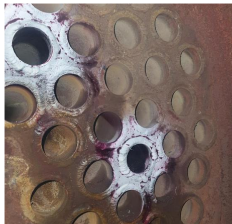
Figure 4. Welded joints of flue pipes after PT techno-economical analysis of repair of flue pipes in steam boiler Oro 65.
