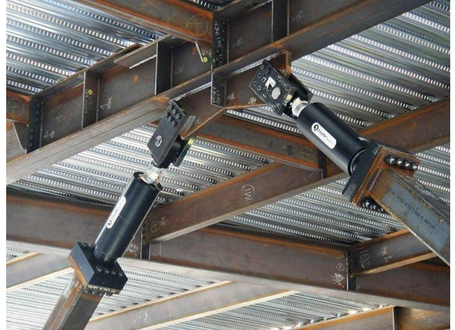
Figure 9. Viscous fluid damper application in steel farm structure.
