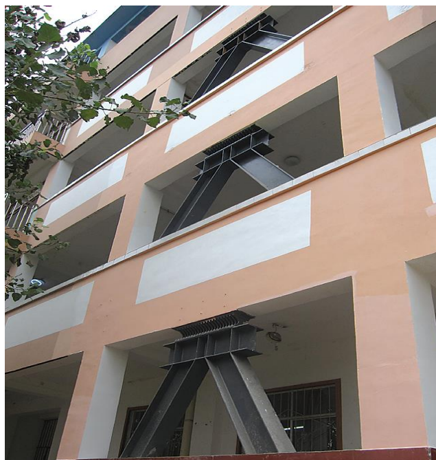
Figure 3. Application of metallic yield damper in a building.
