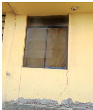
Figure 5. Cracks in walls - house N° 06.
