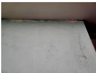
Figure 4. Fissures in walls - house N°10.
