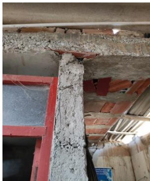
Figure 2. Concrete spalling - house N°12.
