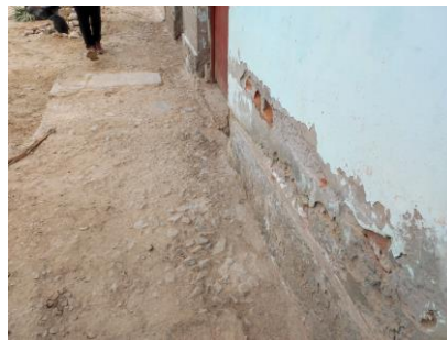
Figure 3. Efflorescence in walls - house N° 06.
