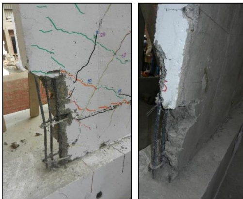
Figure 11. Buckling in reinforcing steel.
