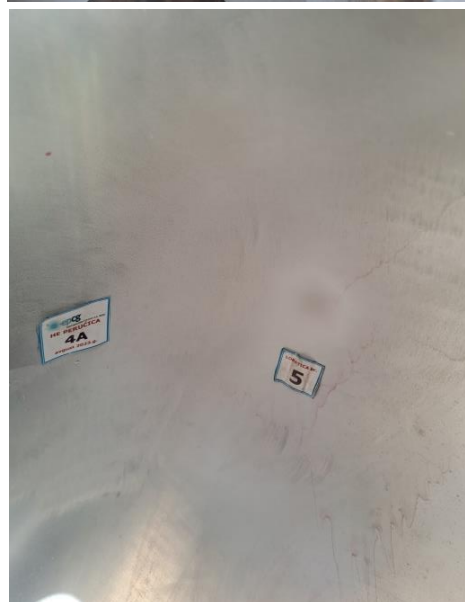
Figure 7. Repaired section of blade no. 5 where the crack was located: top - back side, bottom - front side
