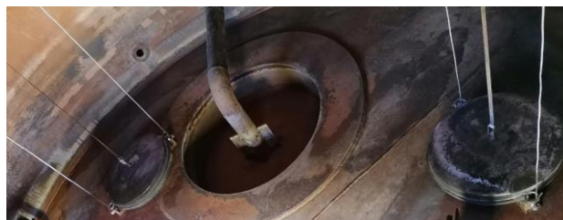
Figure 12. Level gauges in the caustic tank.
