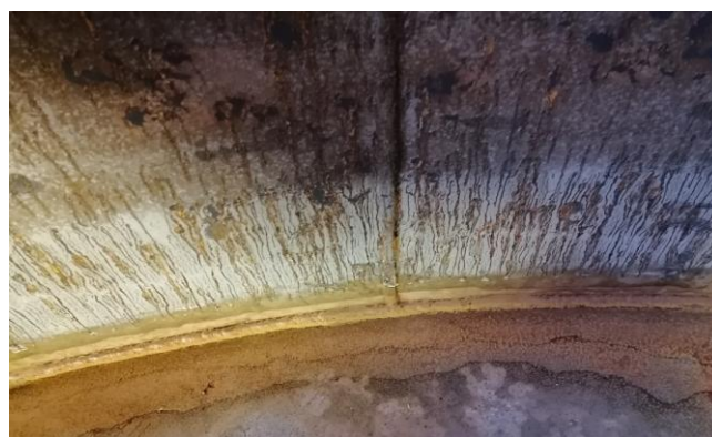
Figure 7. Caustic corrosion observed in the initial phase.
