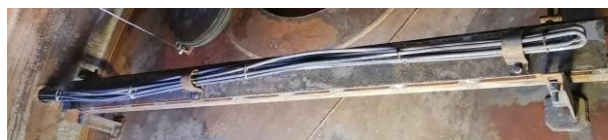
Figure 13. Electric heater found distorted and inoperative.
