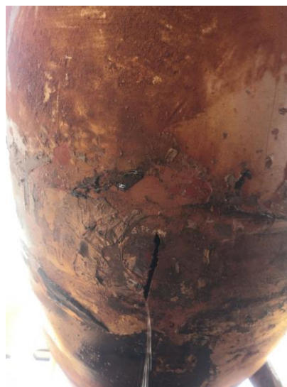
Figure 6. Longitudinal crack in a vertical 20" elbow.
