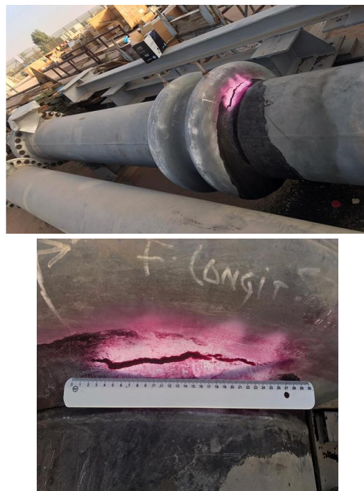
Figure 1. Location of circumferential crack in the expansion joint of heat exchanger.
