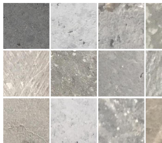
Figure 3. Images of un-cracked condition category.
