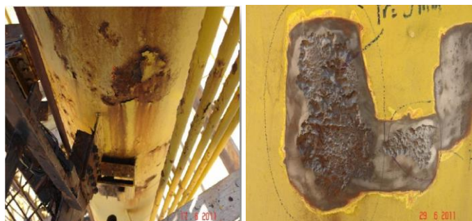
Figure 1. Corrosion of the flare system pipeline (LPG plant).
