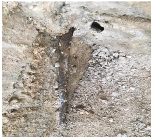
Figure 5. Corroded steel reinforcement bars.
