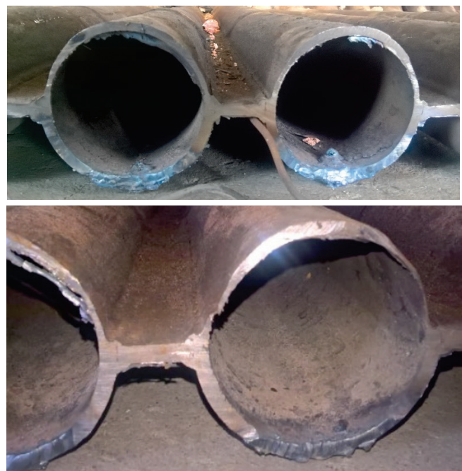
Figure 2. Zones of the largest damage and wall thinning.
