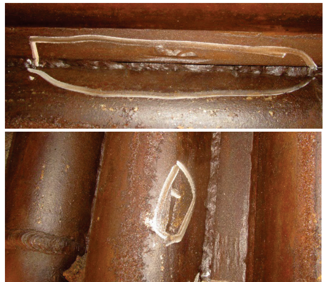
Figure 1. Edge notches in the connection between membrane strips and tubes (top); tube damage (bottom).
