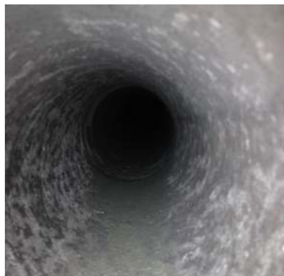
Figure 2. A corroded pipe (top); the same pipe cleaned and prepared by the Tomahawk™ System (bottom). The pipe is clean, dry and ready for liner application, /10/.
