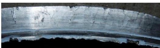
Figure 2. Cracks in the cylindrical part of the austenitic flange neck of a manhole opening, /8/.
