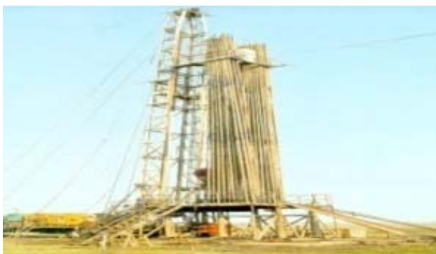
Figure 1. Tower of the repair facilities, /2/. Slika 1. Toranj remontnog postrojenja, /2/
