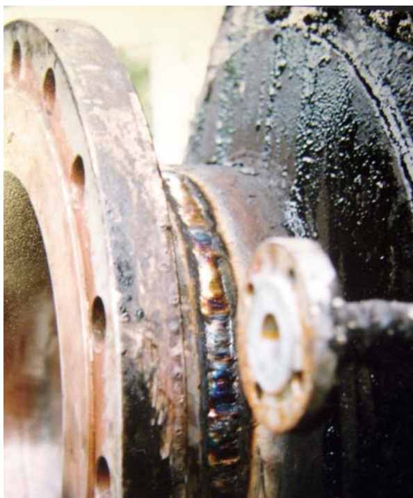
Figure 1. Manhole and welded joint where leakage occurred. Slika 1. Revizionni otvor i zavareni spoj, gde se pojavilo curenje
