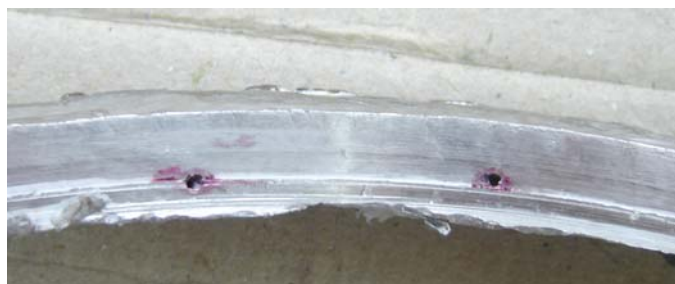
Figure 4. Two pores on inner side of manhole present the initial part of through cracks.
