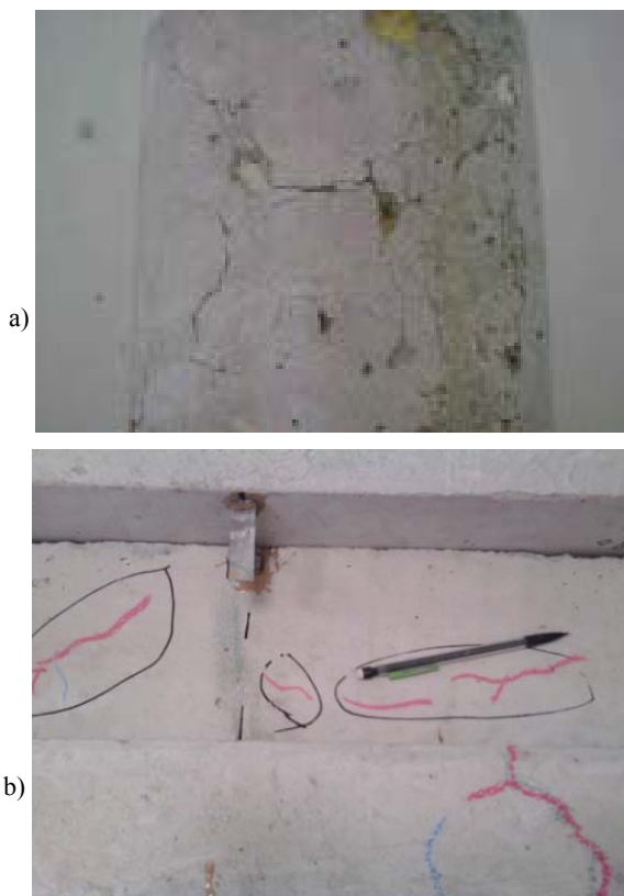
Figure 3. Frost damages specimens after 240 freezing–thawing cycles, a) cylindrical specimen after 240 cycles, b) prismatic specimen after 240 cycles
