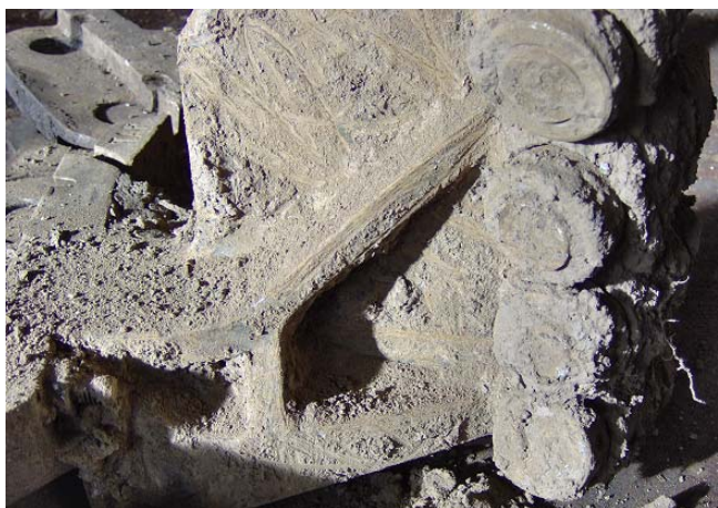
Figure 6. The chain excavator where there are deposits of particles that favour wear. Slika 6. Lančani bager na mestu naslaga čestica koje izazivaju trošenje
