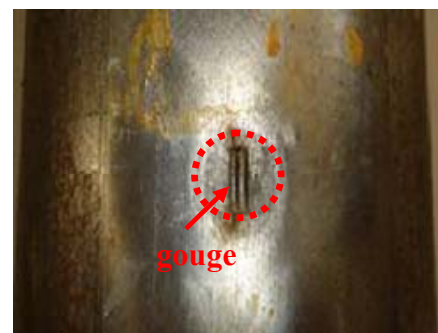
Figure 5. Combined defect of ves. 1 (dent depth \approx 4\% D_e ) after failure. Slika 5. Kombinovana greška pos. 1 (dub. uleg. \approx 4\% D_e ) posle loma
